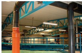
Sewage water treatment plant
